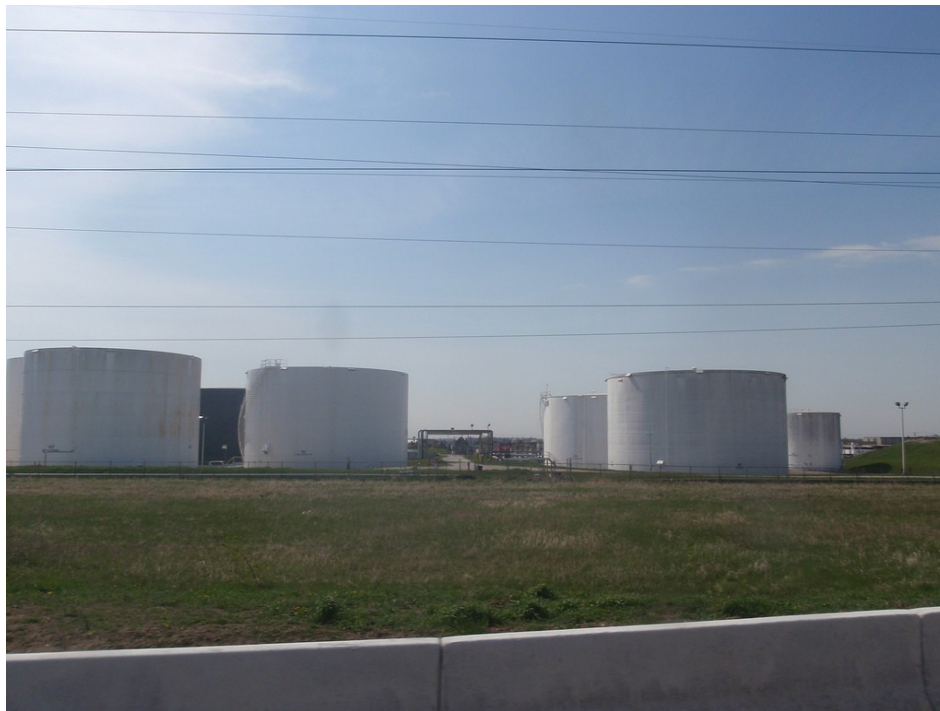
Figure 9.9: You might not know where the tiny town of Cushing, Oklahoma, is. But oil producers and traders around the world do. Cushing is one of the largest oil storage areas in the United States. Storage tanks like these cover more than nine square miles on the outskirts of the town (Davis, 2009). Anthony Easton – More Oil Storage – CC BY 2.0.
